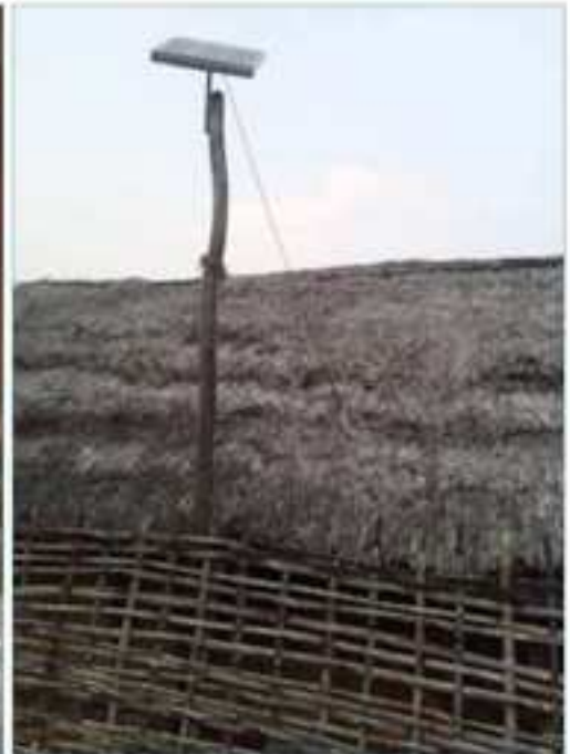
Solar street lights in an unelectrified village
